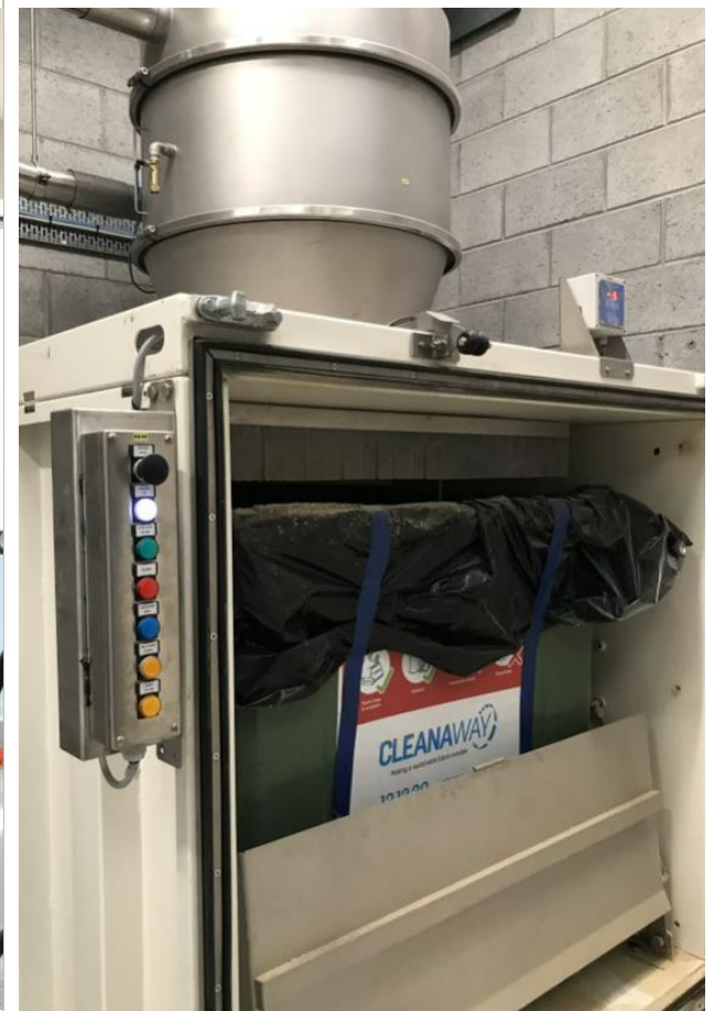
Waste from PC2 zone collected and processed prior to collection
