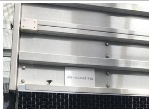
Cooling tower two as labelled – NCC-0211-02
