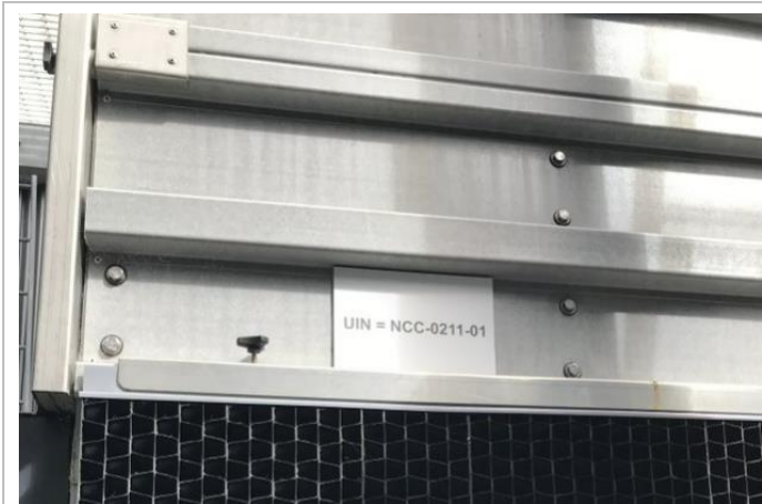
Cooling tower one as labelled – NCC-0211-01
