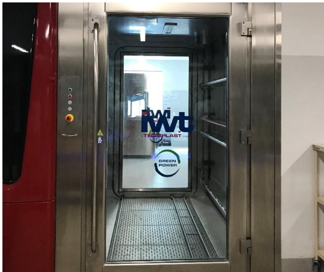
Steriliser in PC2 area secured when not in use
