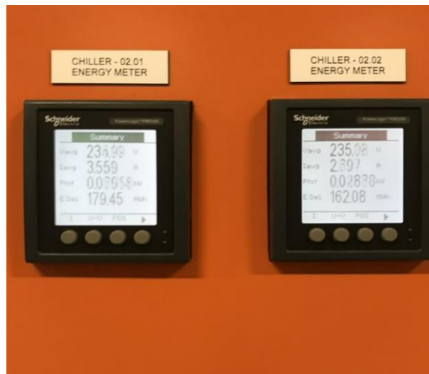
Chillers 02-01 and 02-02 summaries
