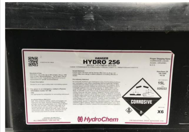
Water treatment chemicals for cooling tower appropriately stored and labelled
