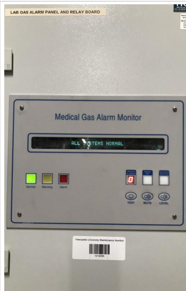
Gas alarm panel and relay board for the laboratory – all systems normal
