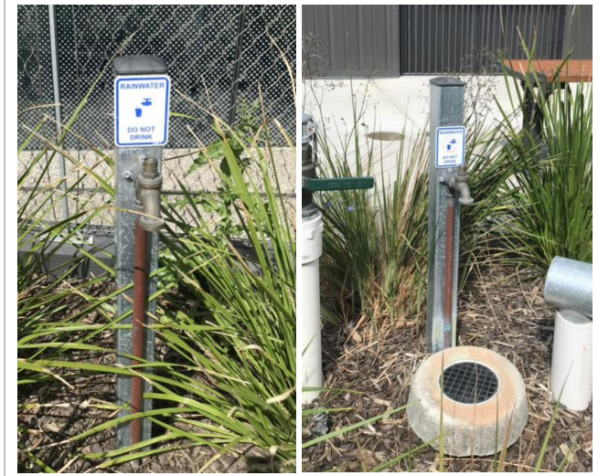
Non-potable drinking water signs installed.
