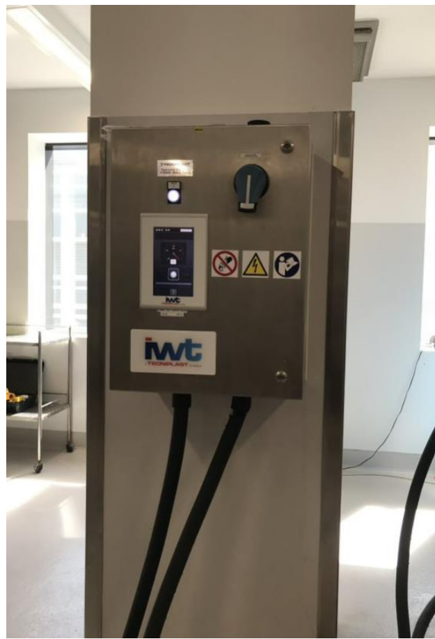
Waste chute and control panel in PC2 zone
