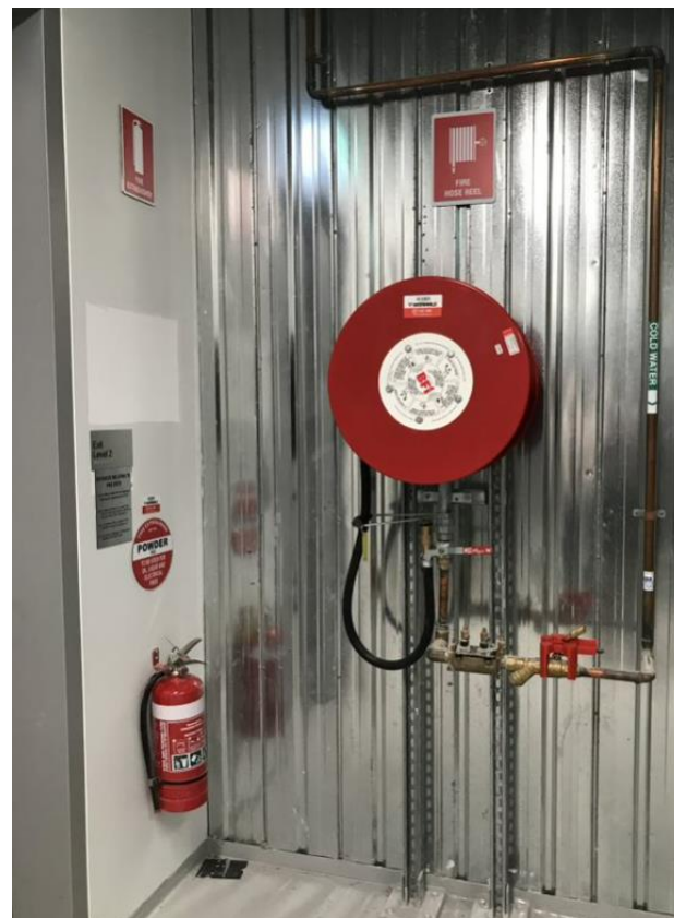
Accessible fire extinguisher and fire hose in plant room
