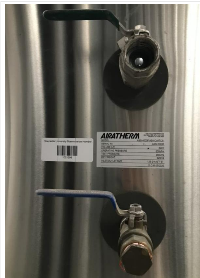
Buffer Tank. Maintenance number is the asset number and visible on all assets.
