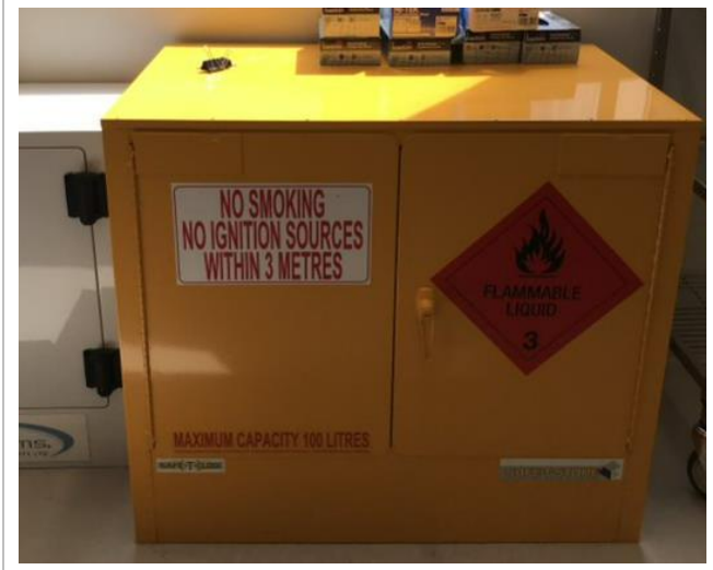
Hazardous substance storage
