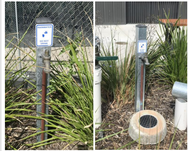
Non-potable drinking water signs installed.
