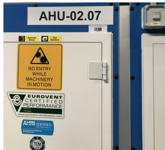
Air Handling Unit (AHU)
