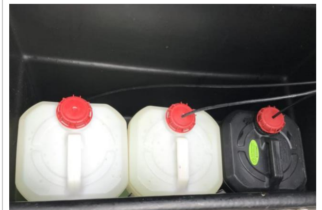
Chemicals inside storage container
