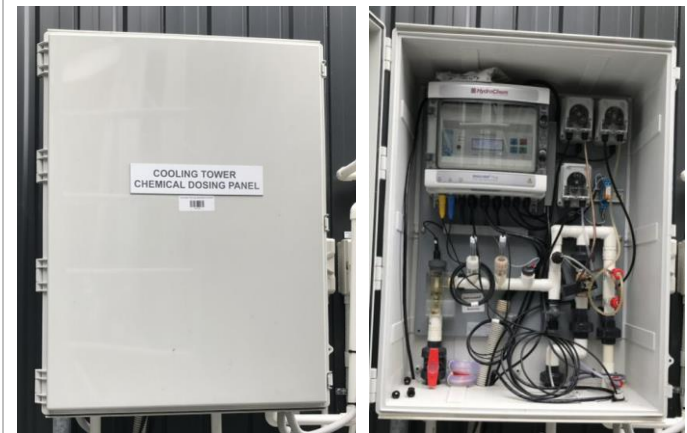
Cooling tower chemical dosing panel secured and suitably accessible for maintenance
