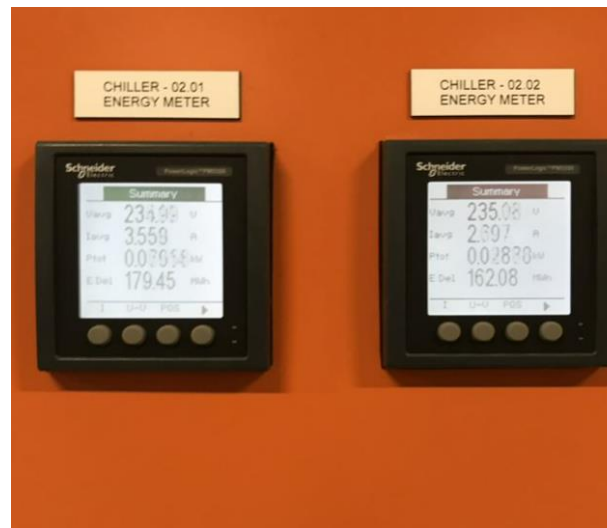
Chillers 02-01 and 02-02 summaries
