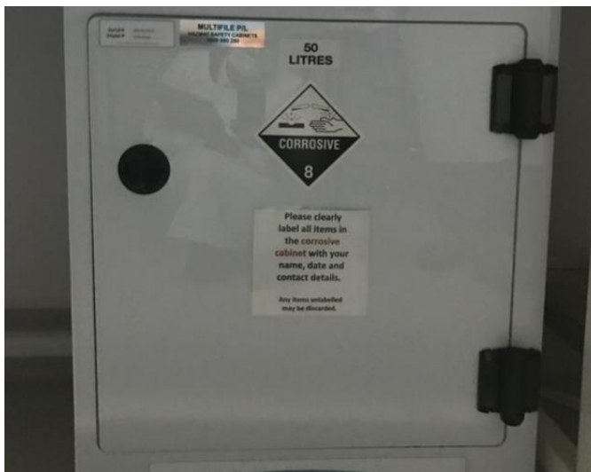
Hazardous substance storage
