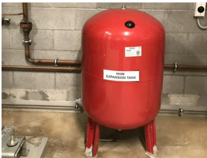
HHW Expansion Tank
