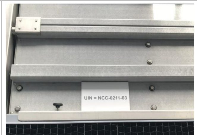
Cooling tower three as labelled – NCC-0211-03
