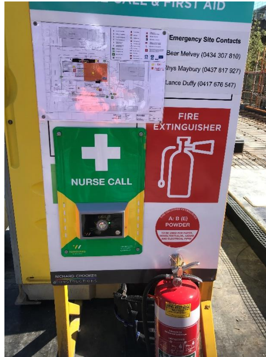
Photo 2 – Emergency response board
