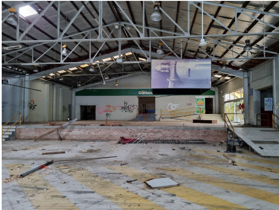
Photo 13: Interior of main structure facing east. Main entrance located behind. Back of the image is top floor and is former area related to historical nursery activities.
