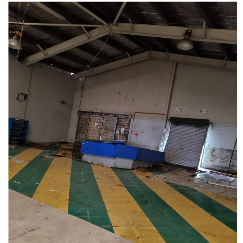
Photo 12: Inside of top floor segment of main structure, adjacent to former nursery area to the east.
