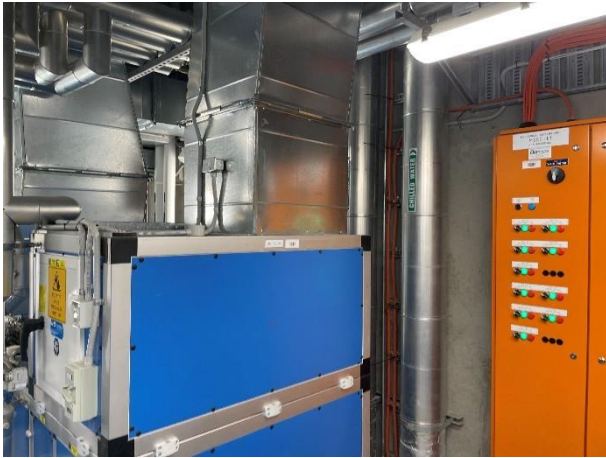
Air handling units and switch board in plant room.
