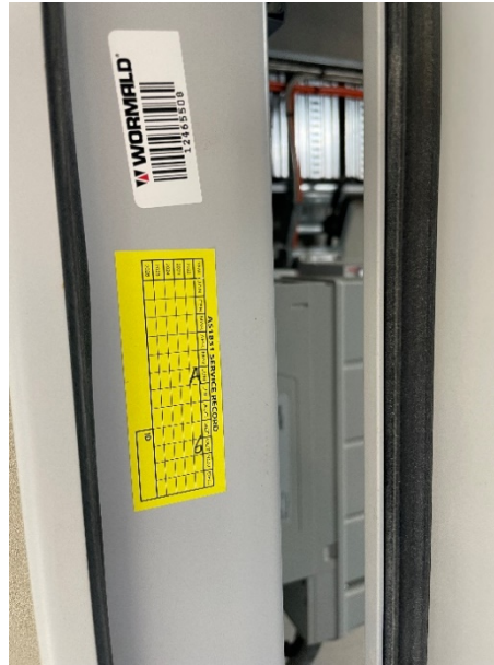
Fire proof door to plant room service tag up to date.
