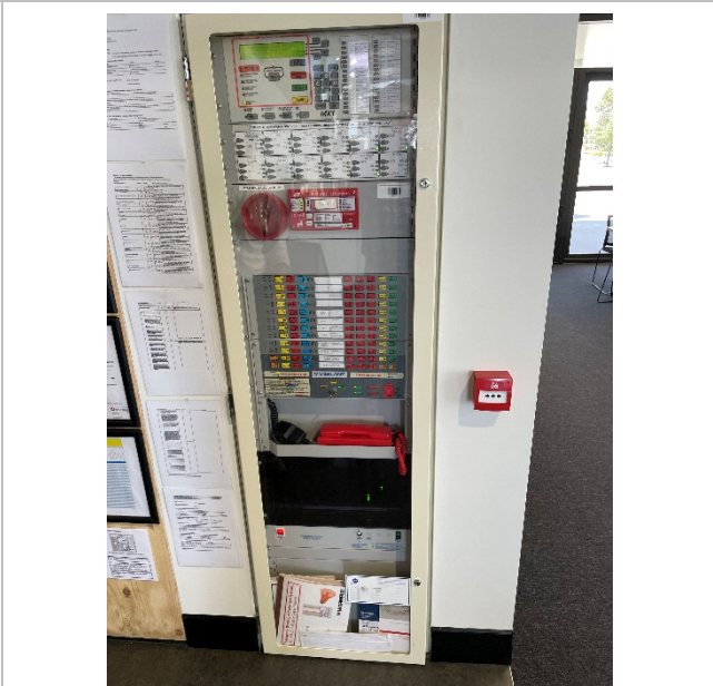
Fire board. Restricted key access.
