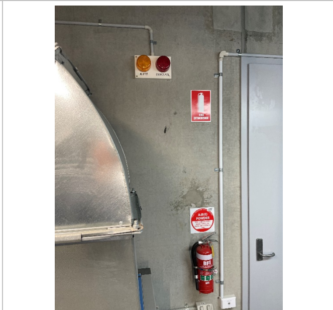
Fire extinguisher in plant room.
