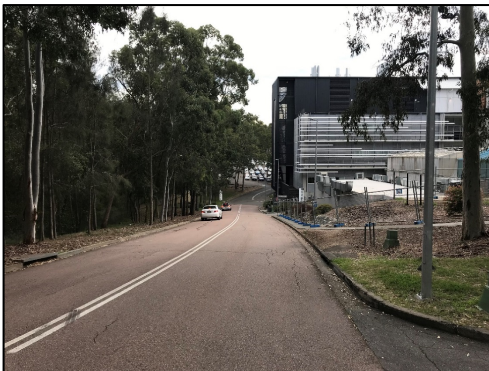
Photo 1 – View north along Ring Road. Construction site to right hand side of the photo
