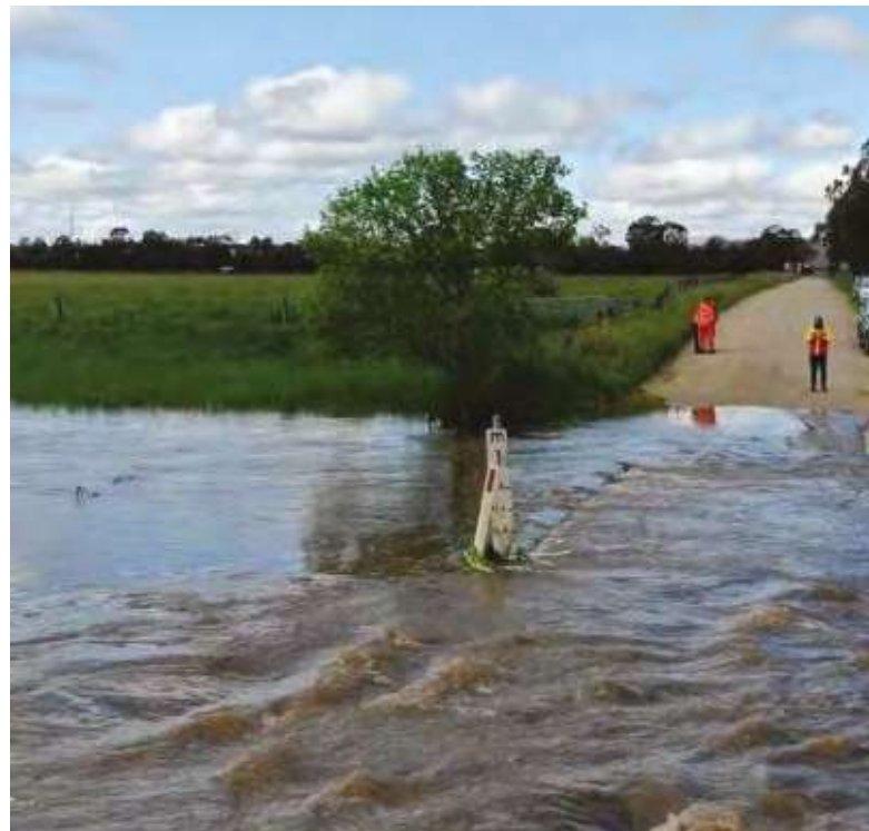
Disruption by floods to the road connection to Aberdeen, Hunter Valley. Image supplied by A/Prof Ifte Ahmed.
