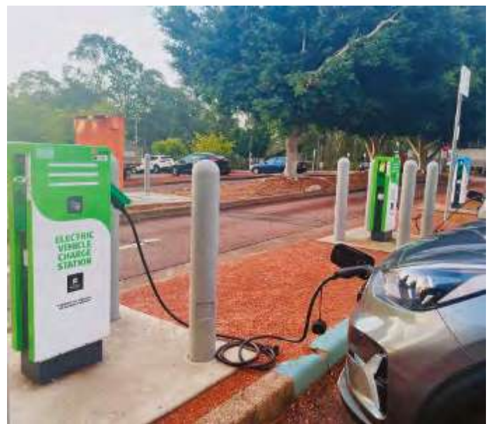
University of Newcastle electric vehicle charging station.
