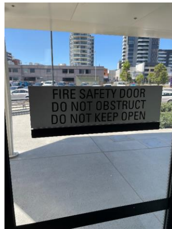
Fire safety door sign.
