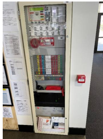
Fire board. Restricted key access.
