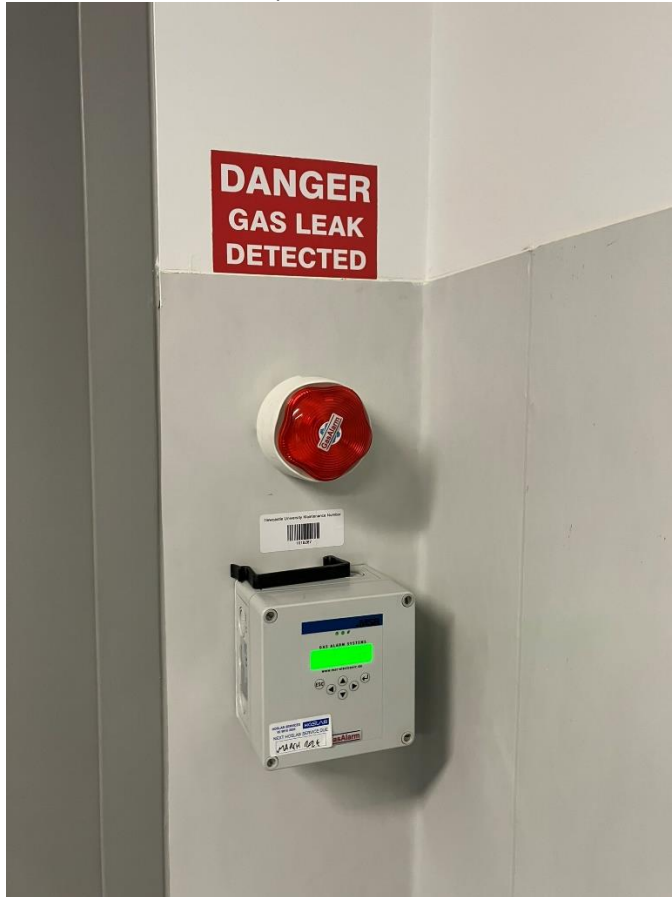
Figure 19 Gas Leak Detector in Operation
