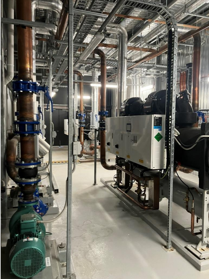
Figure 49 Chiller Room – Plant
