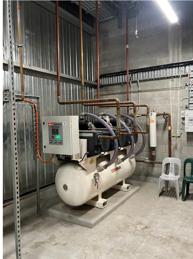
Figure 47 Plant Room – Compressor
