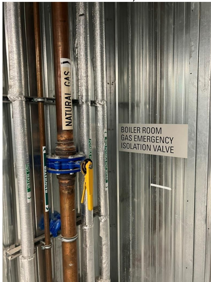
Figure 52 Natural Gas Isolation Valve – Clearly Labelled
