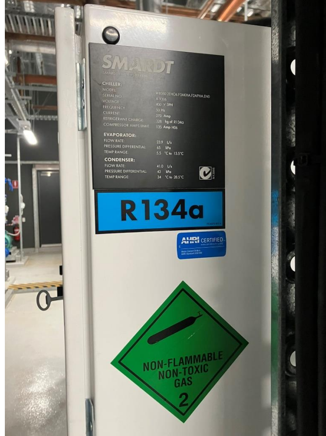
Figure 50 Chiller Room – Control Panel
