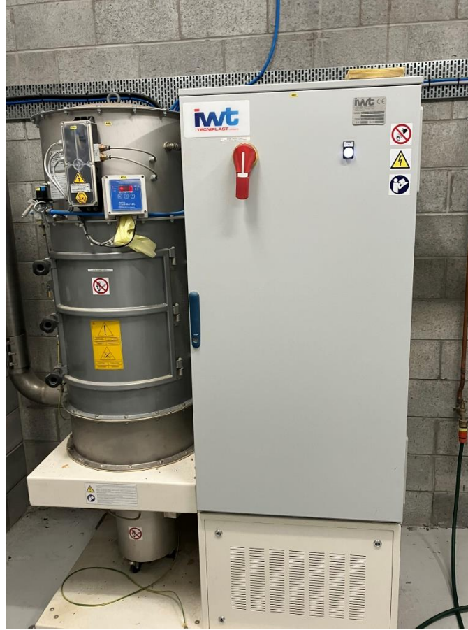
Figure 41 Waste Filtration System (Dust)
