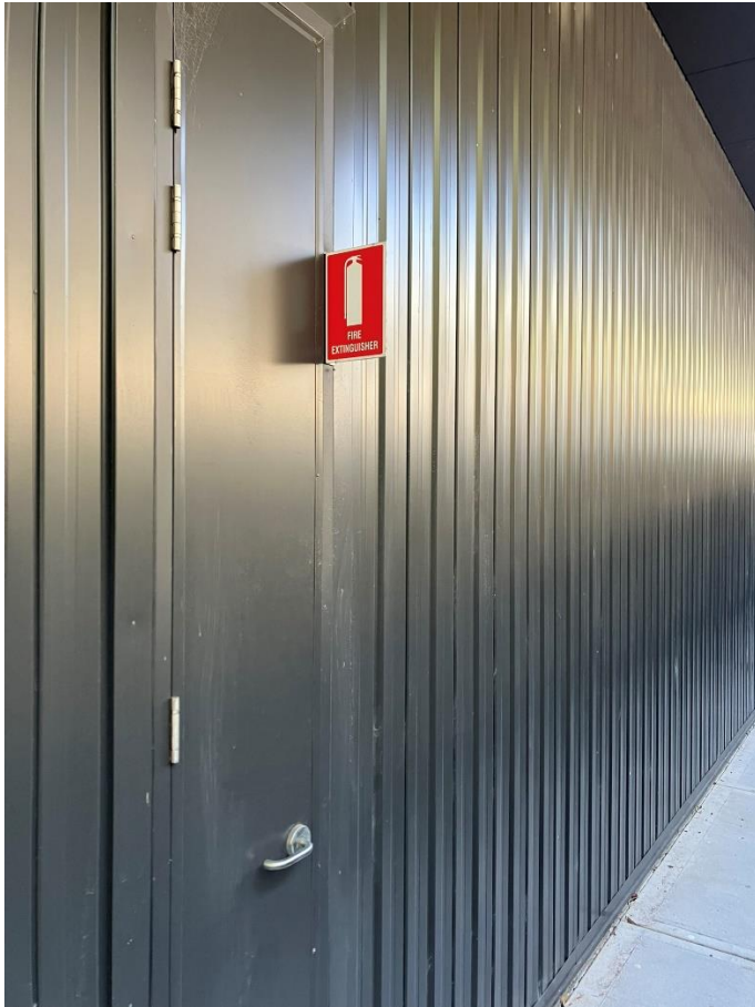
Figure 13 External Signage - Fire Extinguisher
