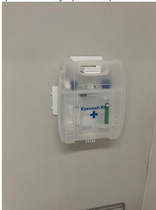
Figure 23 Eyewash Kit in Emergency Shower & Eye Wash Area
