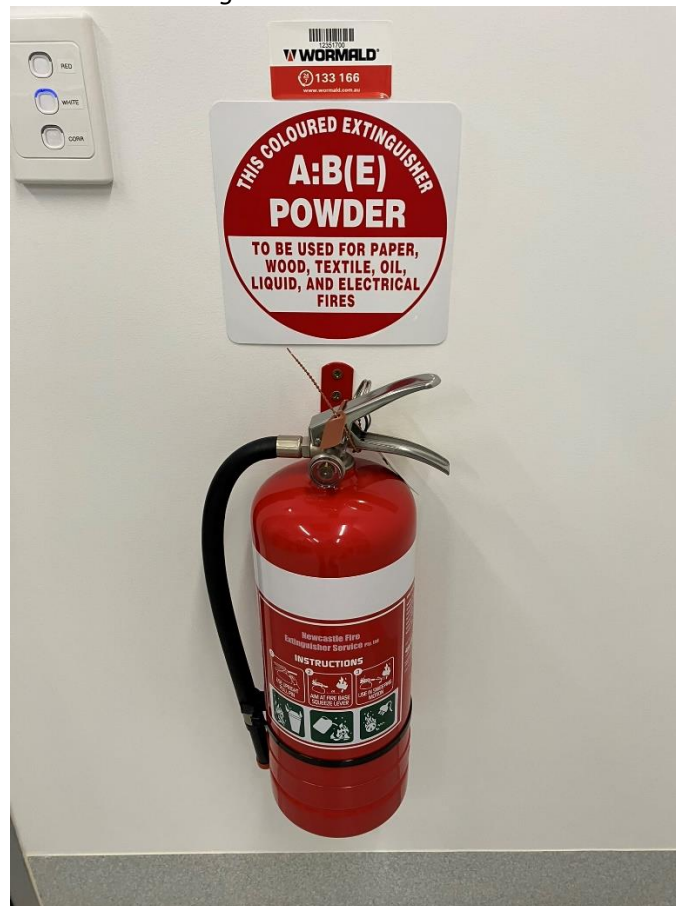
Figure 53 Internal Fire Extinguisher
