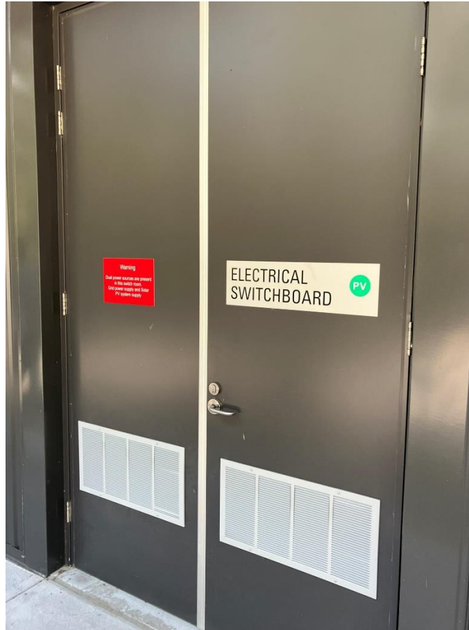
Figure 14 External Signage – Switchboard
