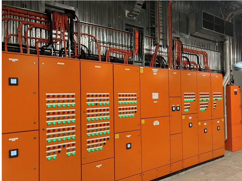
Figure 46 Main Switch Board
