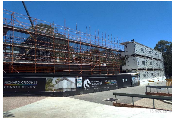
C13 – Evidence of Construction Hoarding
